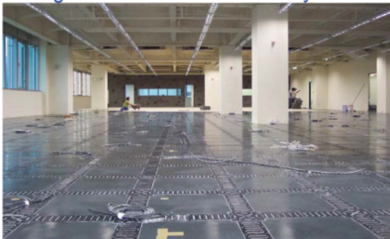
Cables routing inside the Cable Trenches and extending through any point of the interior
