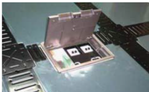
To accommodate large size floor box - Cut at side of the panel (include the Cable Trench width) and install in the trench.
